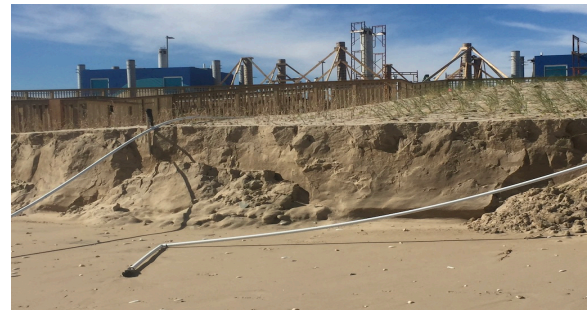
Figure 10. A failed section of restored dune few weeks after construction due to lack of toe protection at South Padre Island, Texas, 2017
